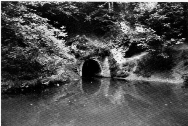
A recent view of the Wrens Nest tunnel portal in Castle Mill Basin.
